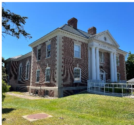
Stone School, Newington (L): This 1920 school has sat vacant since 2003 and was recently condemned. Advocates hope to see the building used for a community center.
