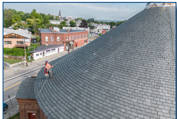
Demolition of the last-of-its-kind Gasholder in Concord was avoided, thanks to our efforts and negotiations with the owner, Liberty Utilities. Our continued leadership facilitated a much-needed stabilization project. Courtesy: William Mitchell
